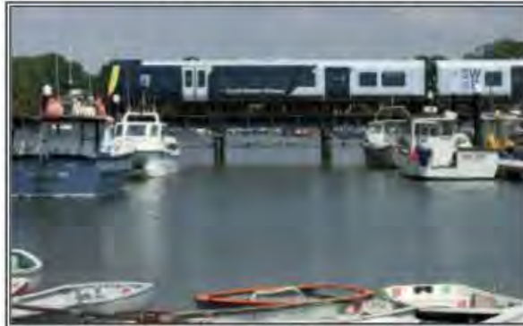
A South Western Railway train crossing the Lyminster River, where work will include improving the durability of the wrought iron columns which support the viaduct
