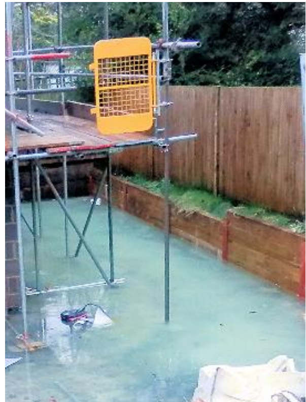
Figure 32: Example of a development in the Littleton district. The building had trenched into the hillside in an area normally dry. The excavation breached the water table in the chalk aquifer during a period of high groundwater.
