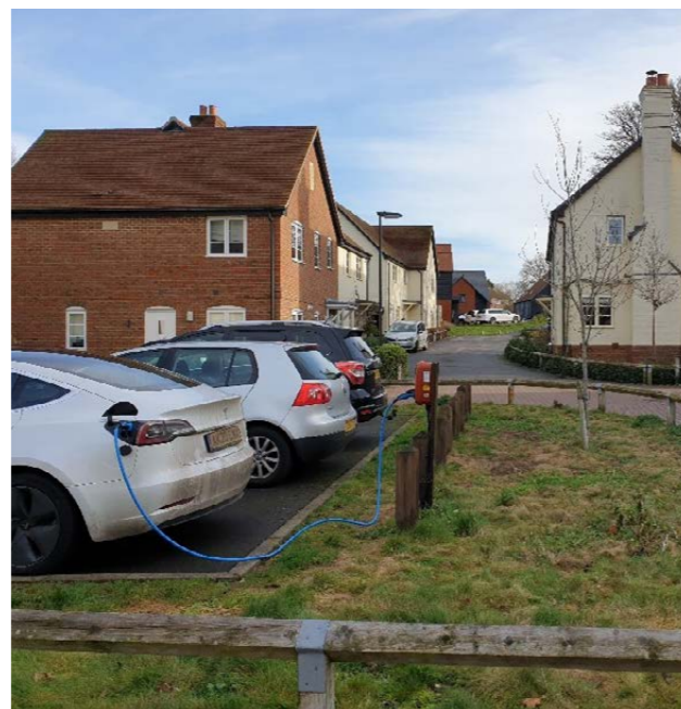
Fig 13: Example of electric car charging points
